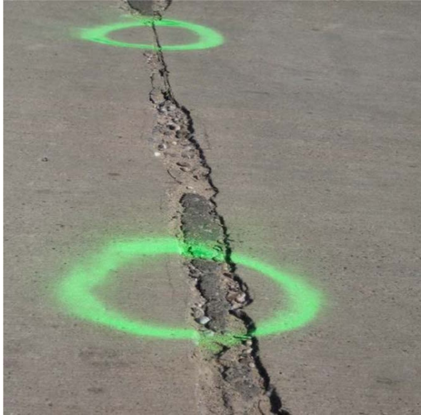
Figure 1. Joint deterioration in Eau Claire, WI (Zhang and Taylor, 2013)
